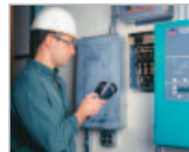
Infrared can accurately and quickly locate faults before failures, shutdowns, or even fires occur.
